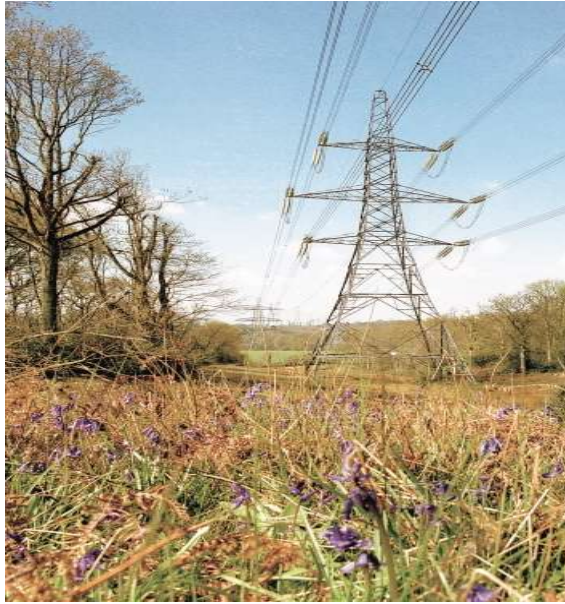
400kV tower and conductors
